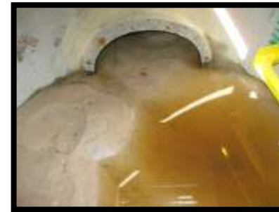
Silt trap and pipe filled with sediment Photo Credit: Swan River Trust
